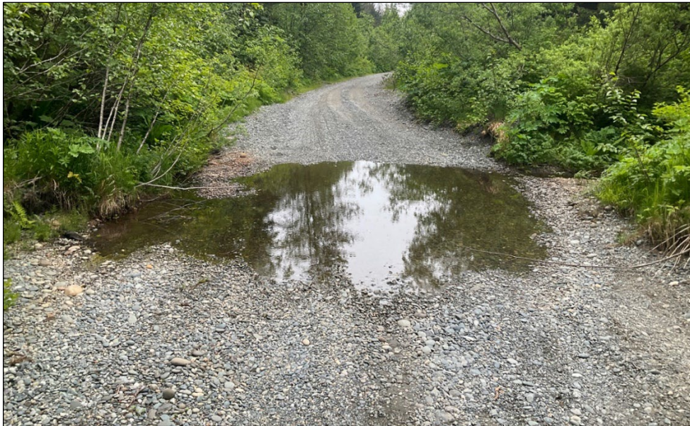
Figure 4.—Water crossing the road at waypoint 266.
